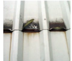
Standard plastisol on hot dip galvanised steel substrate roof after 7 years.
